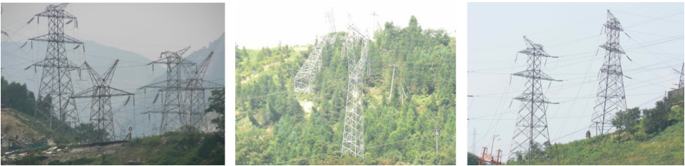
Fig. 1. Pictures of Wenchuan earthquake damage to transmission tower-line system.
